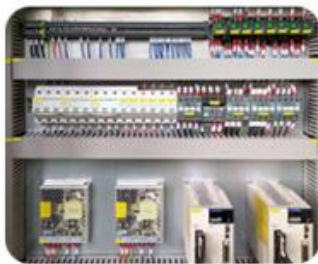
Stable Electrical Cabinet
